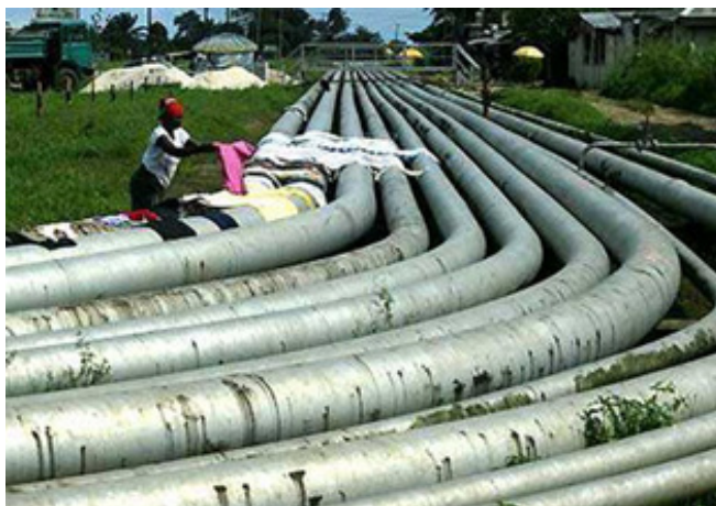
Fig. 3. Poor usage of oil pipeline tracks
